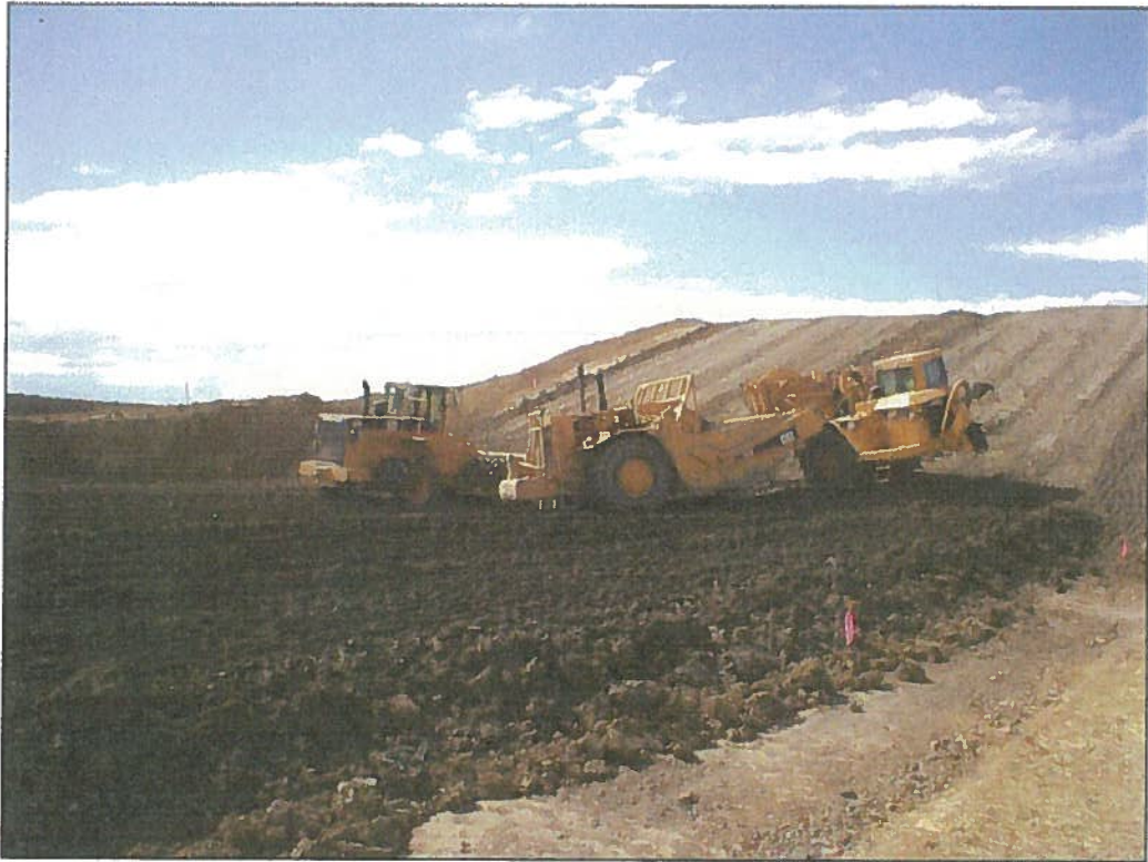
5 - Cat scraper compacting lift 6 on 1.0xE-8 (east side) Test Fill, Cat 815 compacting Lift 7 on 1.0E-7 (west side) Test Fill
