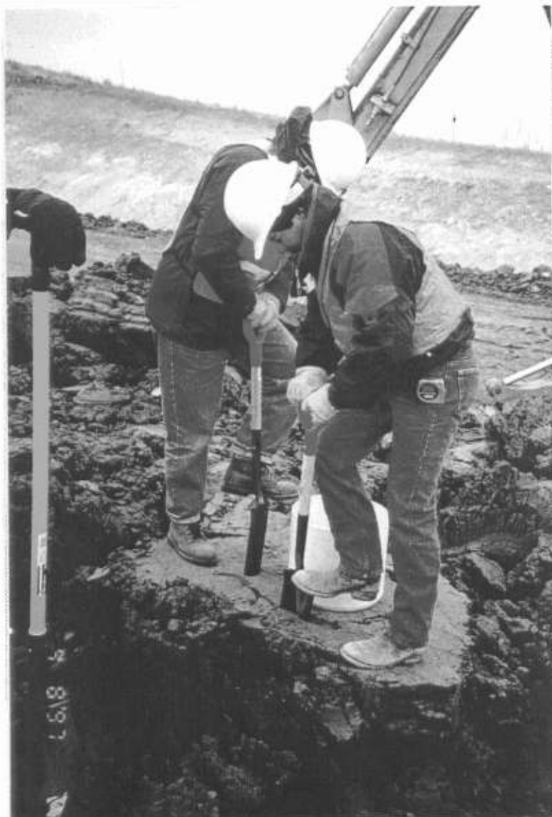
Photo No. 16 Excavation around a block sample location (area beneath ring in center of photograph). The backhoe in the back- ground was used to excavate the trench around the sample location.
