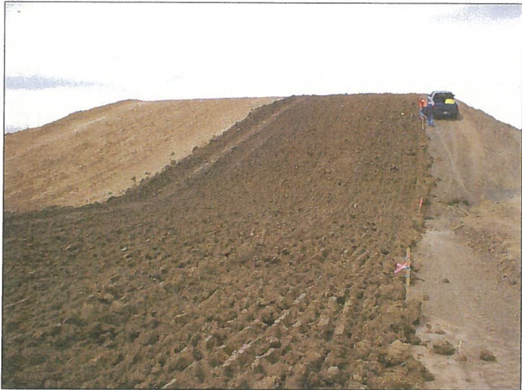
3 - Testing first lift on the east side of the Test Fill (Cat 815)
